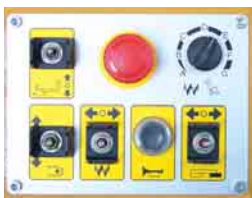
Left-side main screed control panel
